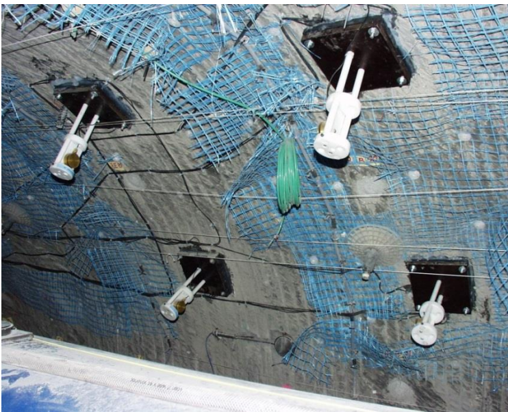
Fig. 2.5 Details of the seismic instrumentation. Four transducers located in the later backfill.
