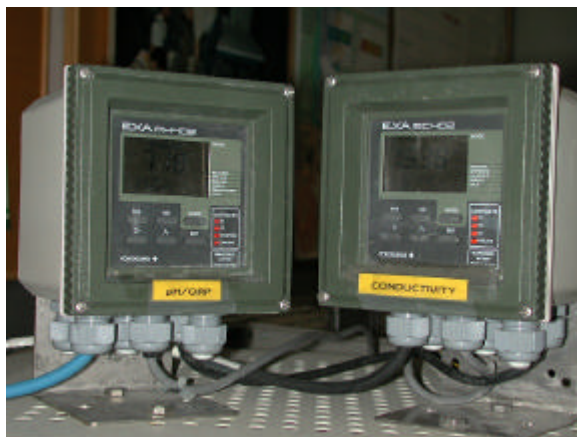
Figure 3-6: Yokogawa GCh transmitters installed on the DAS 19"-rack.
