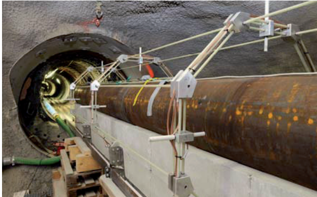
Figure 2. Construction of the instrumentation and liner modules at the microtunnel mouth (Picture Comet Photoshopping GmbH)
