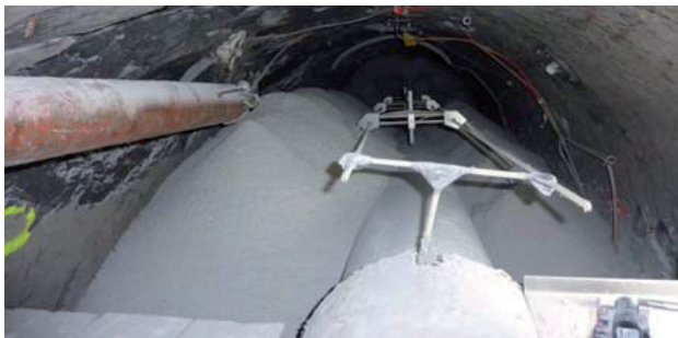
Figure 3. HE-E construction: emplacement of the MX80 pellets in the microtunnel in the Opalinus Clay at Mont Terri using the auger technique (Picture Comet Photoshopping GmbH).
