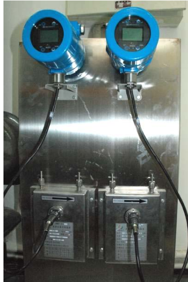
Fig. 15 Coriolis-based mass flowmeters.
