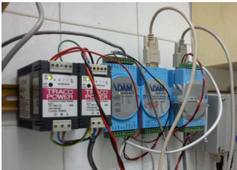
Figure 15: Data acquisition modules and their power supply
