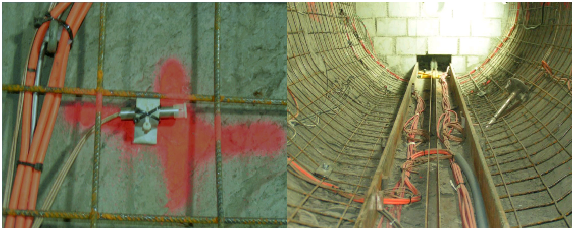
Fig. 6.9: Installation of the humidity sensors (left) and emplacement of the cables in the cable shaft (right).
