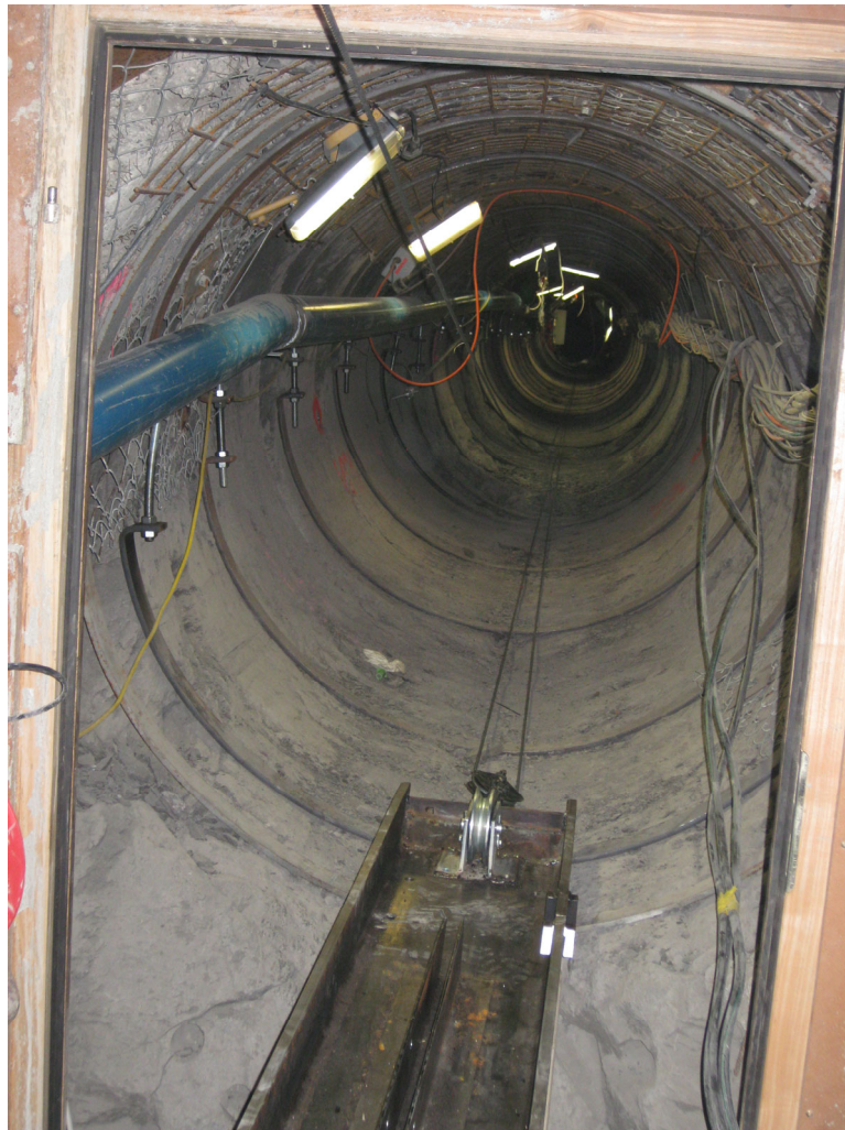
Fig. 2.12: Installation of the railway system into the microtunnel thanks to a pulley-winch system.
