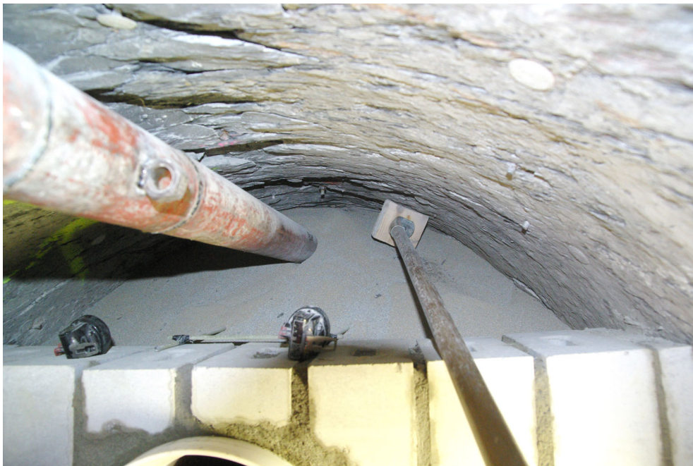
Fig. 6.25: Sand/bentonite section shortly before finishing backfilling. On the right: Shuffle for filling the roof gap.
