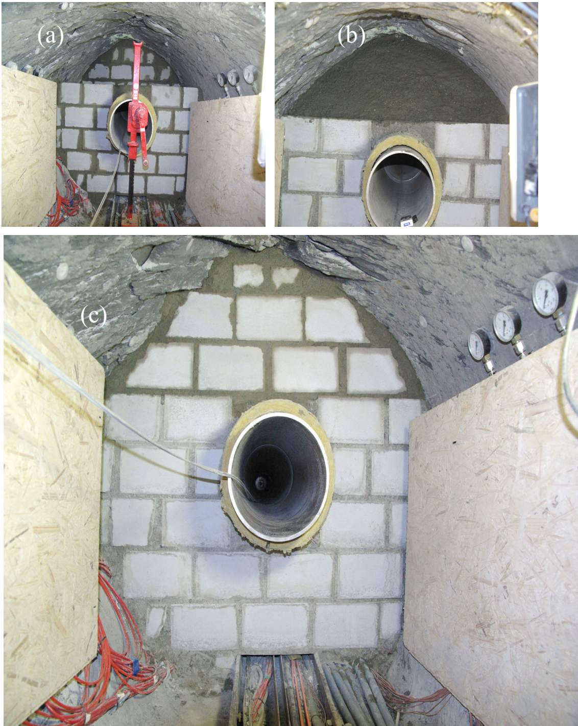
Fig. 6.7: Plug #3: (a) dying end scaffolding wall for concrete block; (b) concrete block; (c) last wall as completed.
