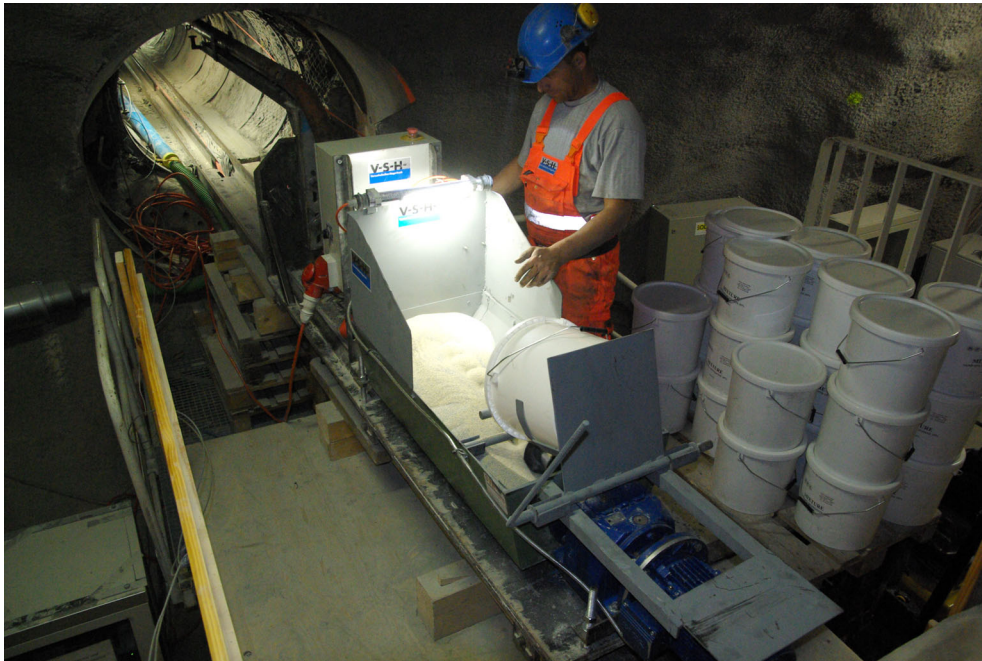
Fig. 6.22: Sand/bentonite filling equipment.
