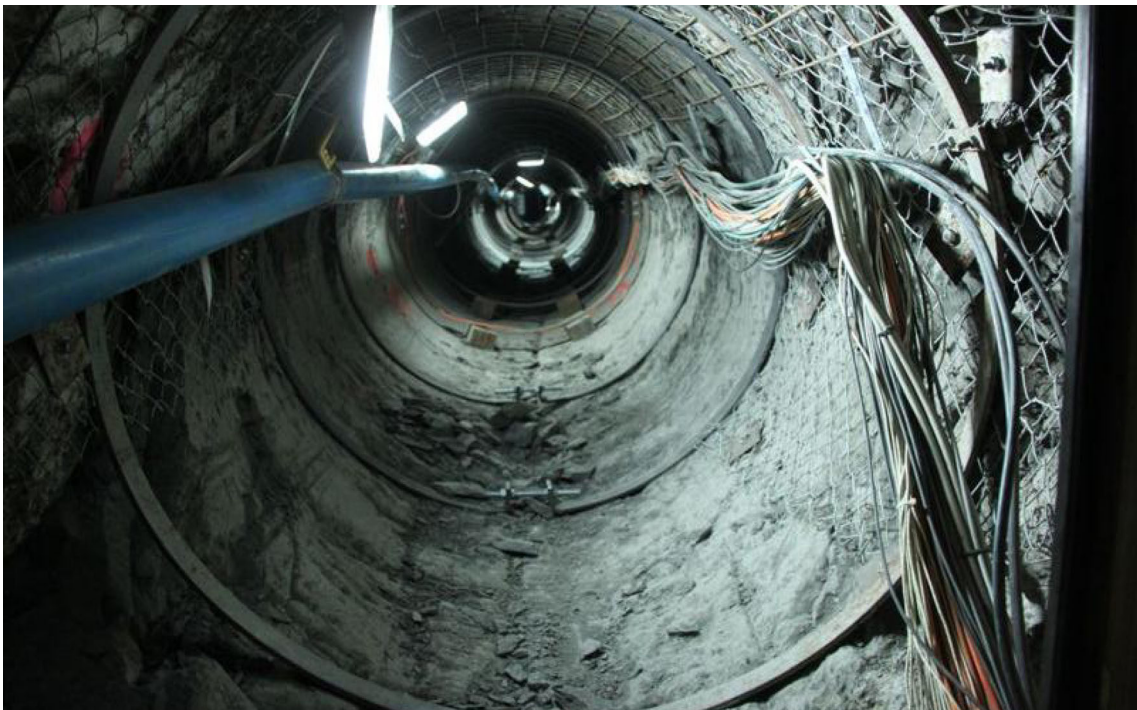
Fig. 2.10: Replacement of the steel rings (those in front have been replaced) to permit the emplacement of the railway system (picture from Swisstopo).
