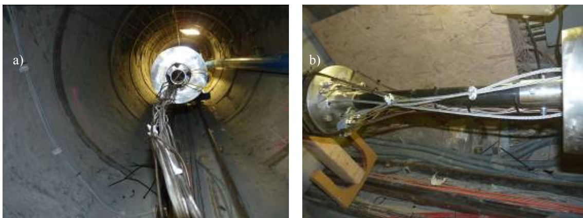
Fig. 6.32: a) Cables from heater 2 entering in heater 1. b) Detail of the PPS tube connecting heater 1 and heater 2.
