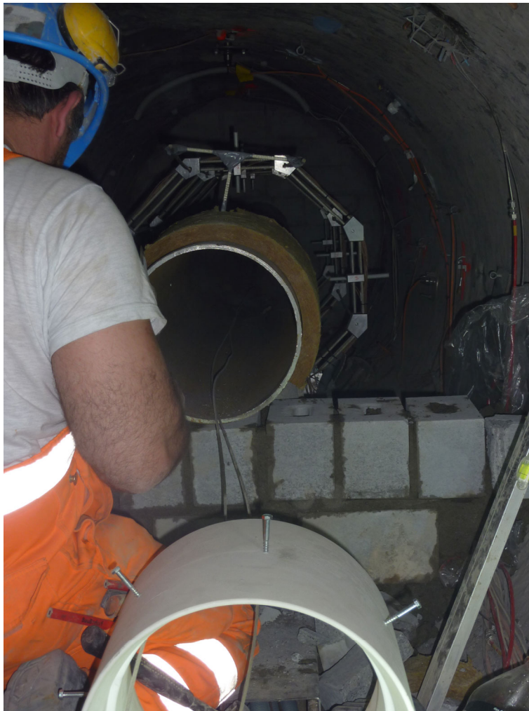
Fig. 6.15: Construction of the first wall of plug #2 as fixed support of the liner.
