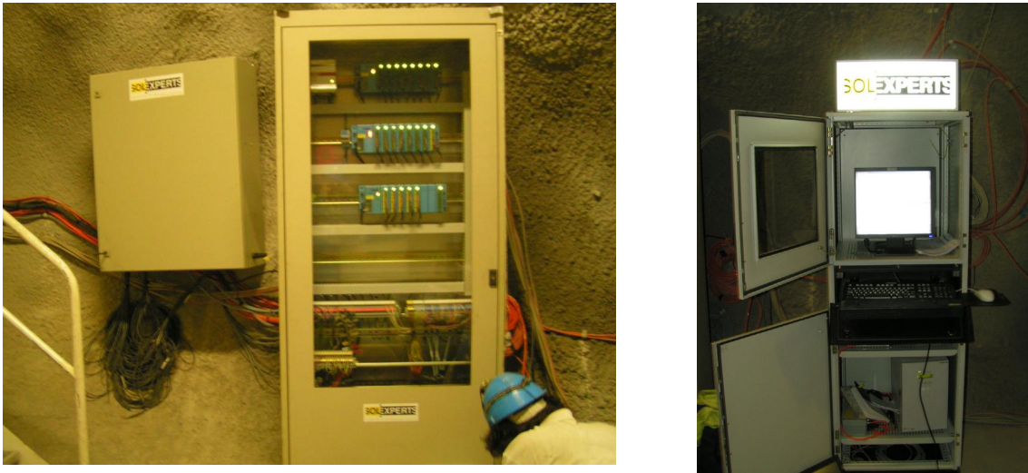
Fig. 6.8: Renovated module rack and read-out rack for the humidity sensors (left); PC rack for the Geomonitor (right).
