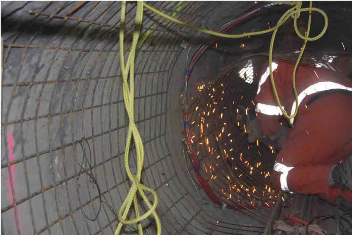
Fig. 2.16: Emplacement of temporary steel nets (picture from Swisstopo)
