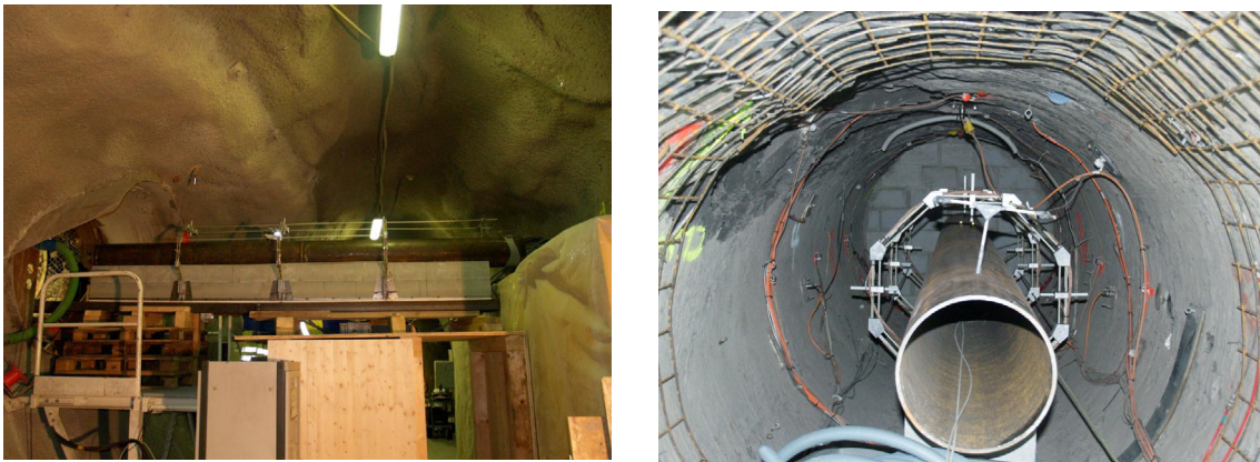
Fig. 6.11: Completed Nagra modules on the platform (left) and after towing in the microtunnel.
