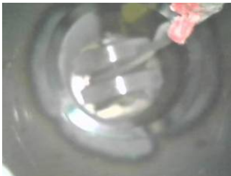
Fig. 6.36: Detailed of the pulley and the twisted traction cable.
