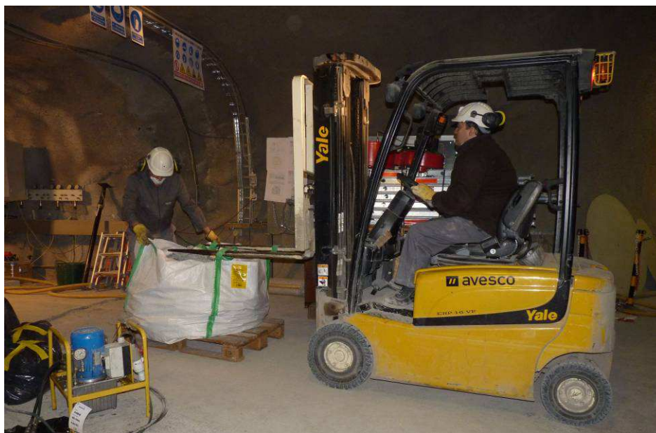
Figure 15: Loading forklift with debris
