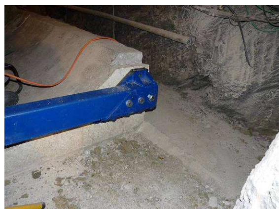
Attachment of the lateral part of the metallic beam to the concrete bed
