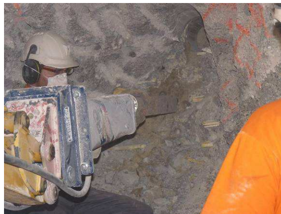
Pushing the sampling pipe with the help of the backhoe into the bentonite
