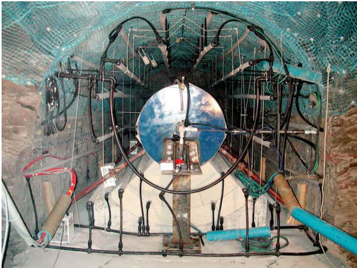
Figure 2: Appearance of the concrete and bentonite blocks bed, dummy canister and hydration system before the installation of the GBM (ENRESA 2005)
