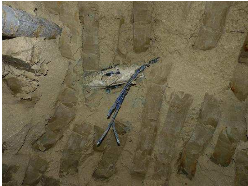
Figure 69: Broken cables during the bentonite removal
