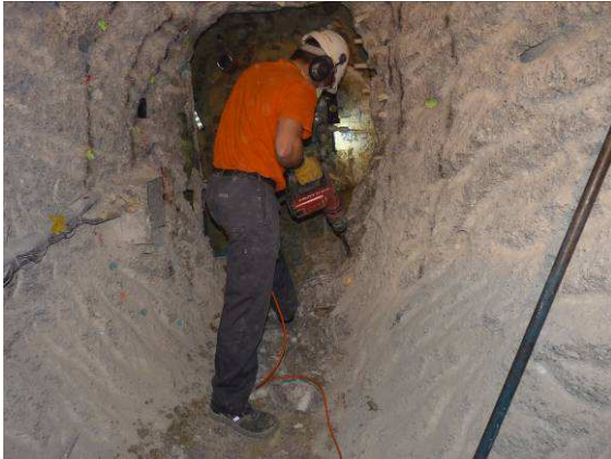
Use of hand tools to remove the concrete plug after the effect of the expansive cement (I)
