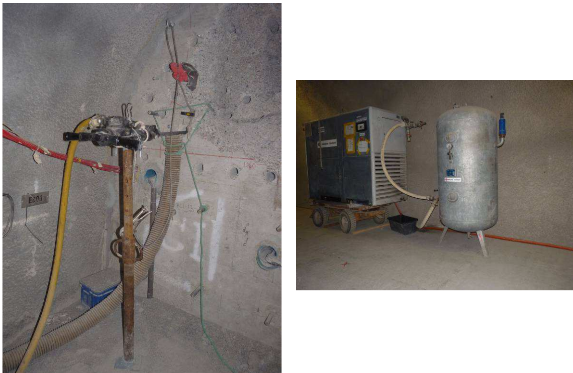
Figure 11: Pneumatic hammer and compressor (left/right)
