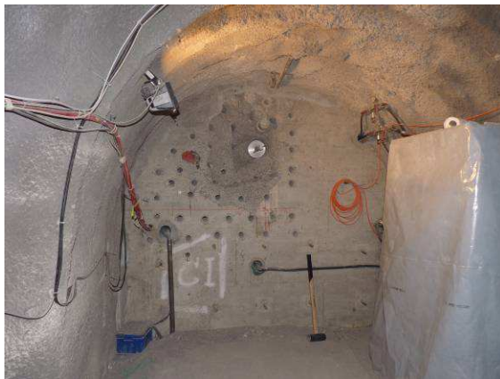
Holes around the main opening in the plug
