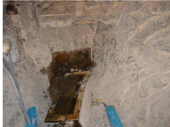
Cable box C dismantling (III). Water spot
