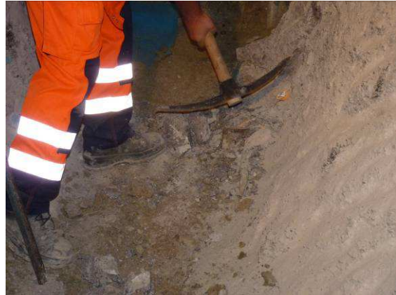
Use of hand tools to remove the concrete plug after the effect of the expansive cement (II)
